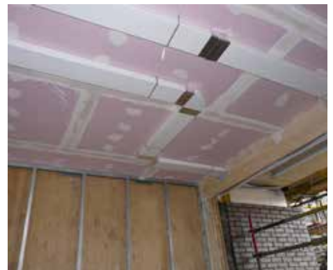
Building systems are routed through a ceiling void created with gypsum board. Photo credit: Willmott Dixon Group
