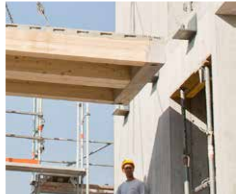
Angled steel brackets connect hybrid floor slabs to concrete access core. Photo Credit: www.creebuildings.com
