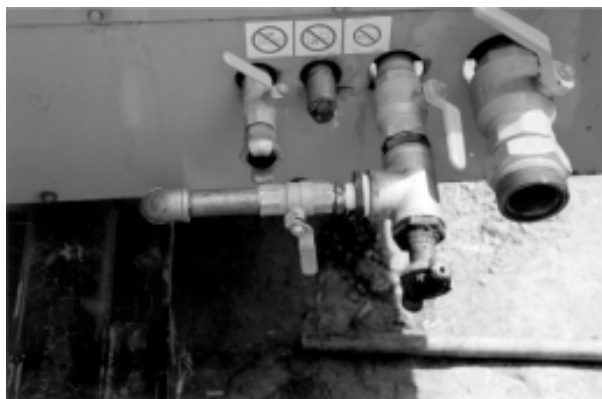
Figure 7.11 Air development manifold – Allowing discharge to atmosphere
